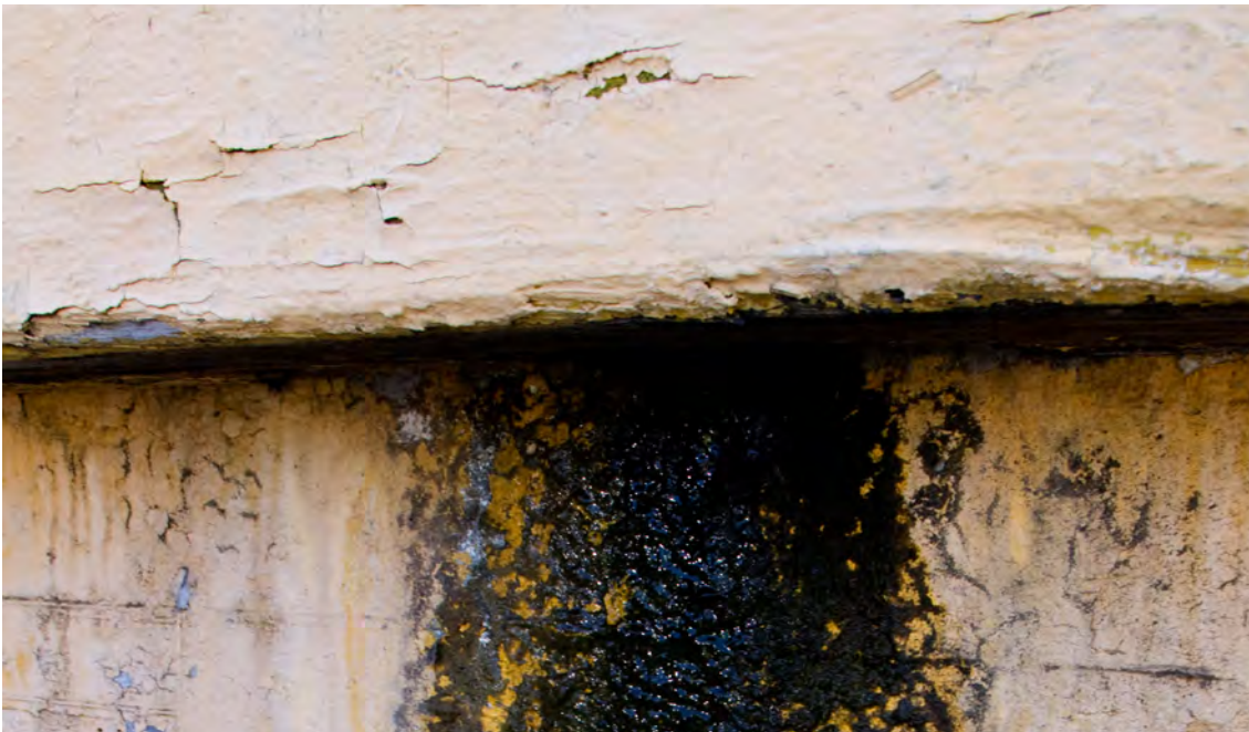
Fig. 1: Water damage. Photo credit: zo-jo.
