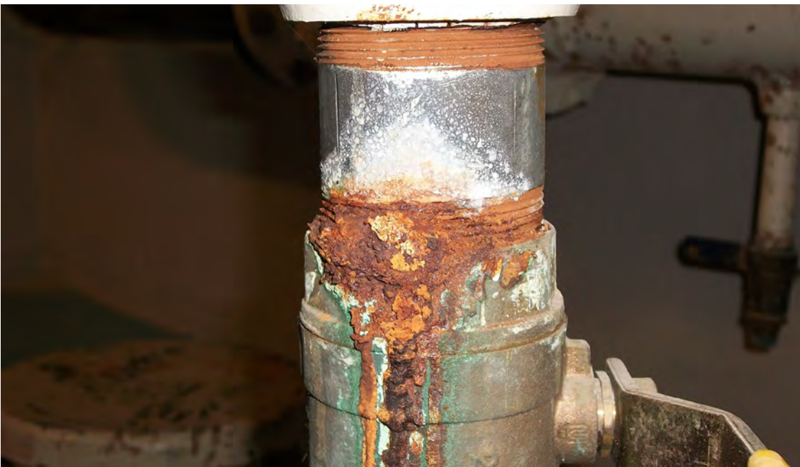
Figure 3: A busted pipe. Photo credit: Corrviv.
