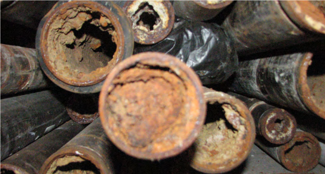
Figure 2: A rust-clogged pipe. Photo credit: Corrviv.
