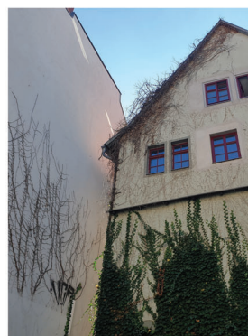
Scratched wall by the plant
