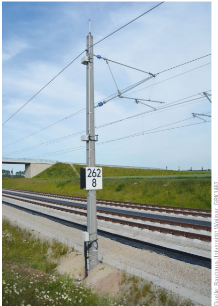
Bild 1 Schleuderbetonoberleitungsmast entlang der ICE-Neubaustrecke Spun cast reinforced concrete pole at the high-speed railway track
