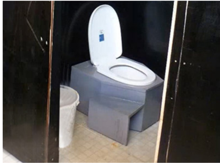
fig. 2.11: example of a dry toilet. ClimEtSan. (Prost 11/13/2020)
