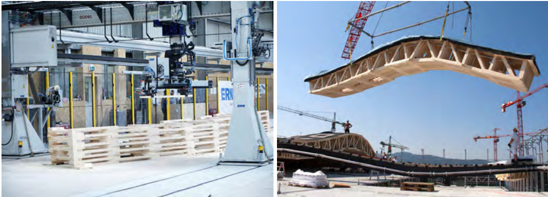
Figure 2.4: Fabrication of the “Sequential Roof”. Left: Placement of a part at its destination position. Right: Installation of a pair of partially pre-fitted trusses on site. Photographs by Aleksandra Anna Apolinarska, 2018.
